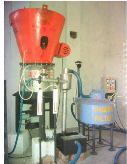
Biomass Gasifier installed at Karansinghji Ki Khedi
