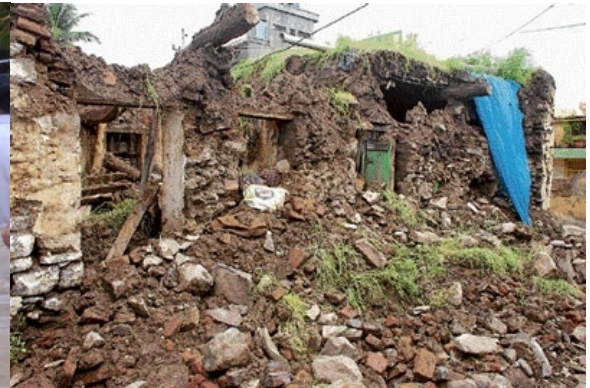
House in Bijapur, Karnataka collapses due to incessant rain (www.deccanherald.com)
